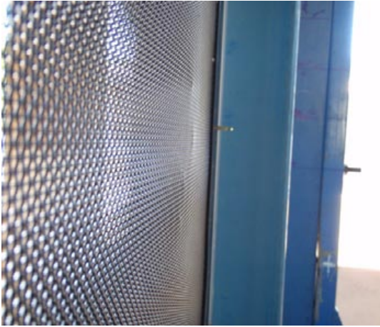
Figure 3: Inside view of typical damage after Trial S1.1
